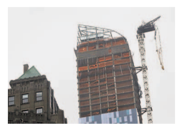
WEST 57TH STREET A broken crane at a construction site.
