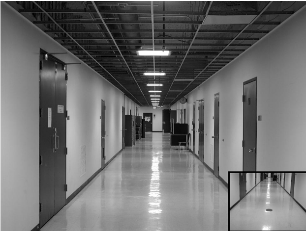
Figure 2: A photograph of the real hallway, with a scaled inset of a screen shot looking down at the target
